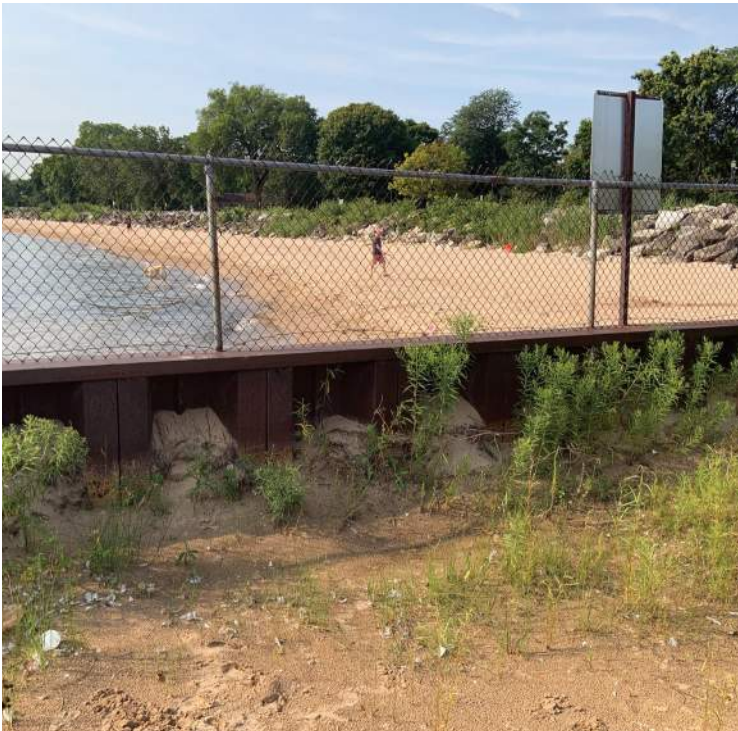
VIEW OF EXISTING GROIN WALL, LOOKING SOUTH FROM CLARK STREET BEACH, WITH DOG BEACH IN THE BACKGROUND
