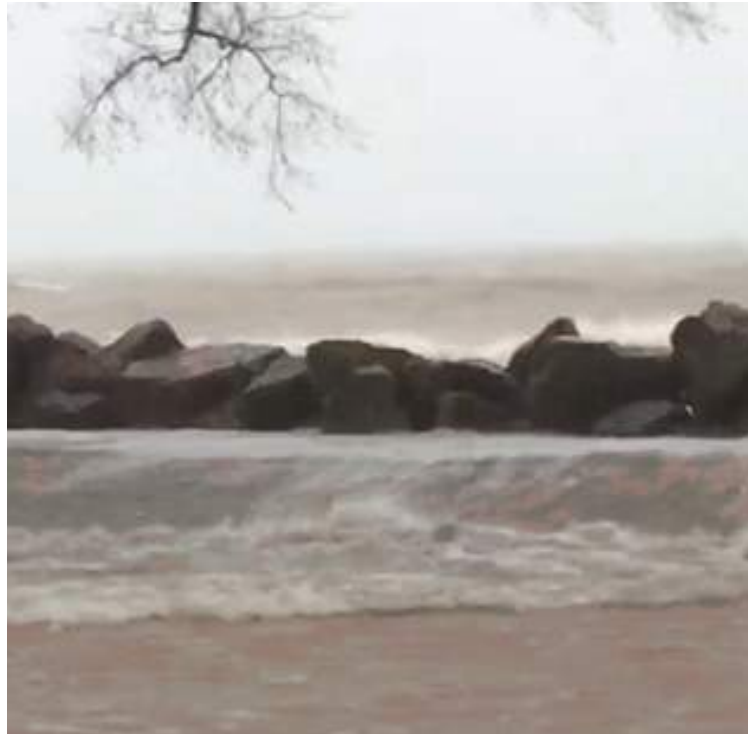
FLOODING AT CLARK SQUARE PARK CAUSED BY OVERTOPPING OF THE REVETMENT DURING 2020 STORM
