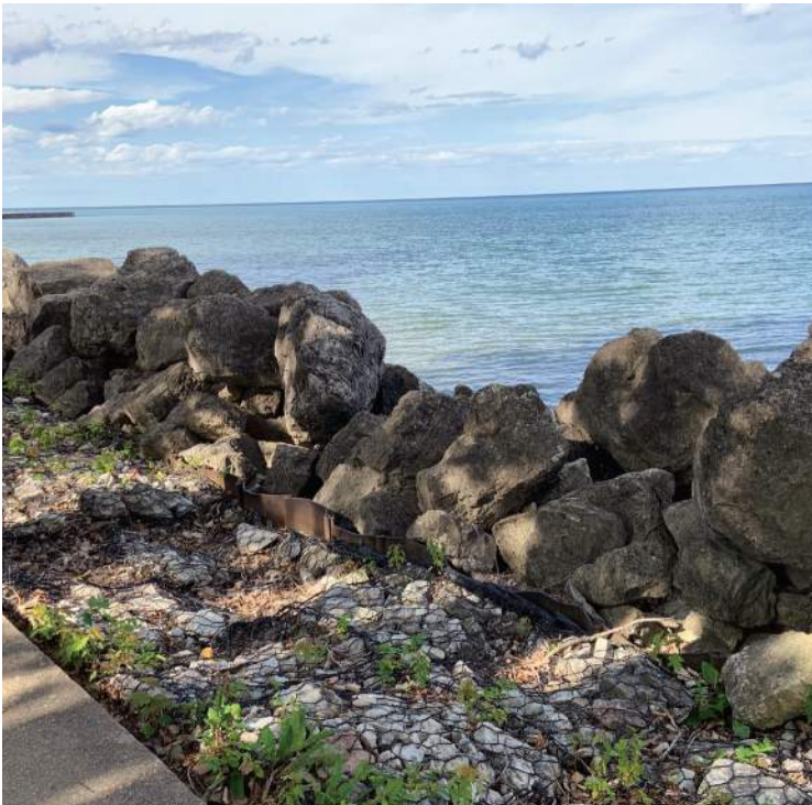
CLOSE UP VIEW OF THE REVETMENT MATERIALS, WITH GABIONS, SHEET PILE AND RUBBLEMOUND ALL VISIBLE
